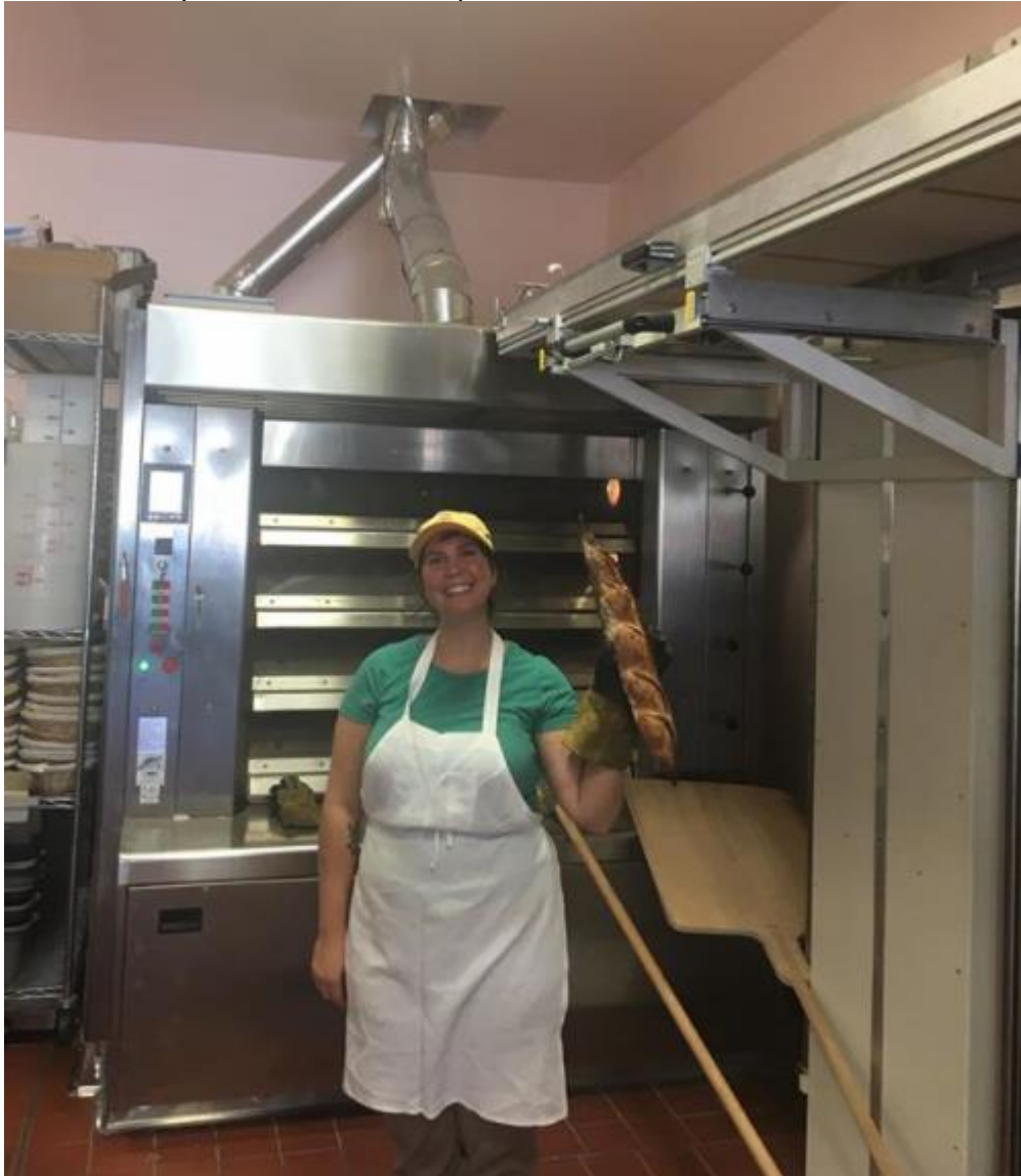
Photo: Iliana Berkowitz, owner As Kneaded Bakery, San Leandro, CA TMB Baking Stoneheart/Bassanina Tubix 420-D (1.6M deep x 1.2M wide, 2 doors) with tower loader
