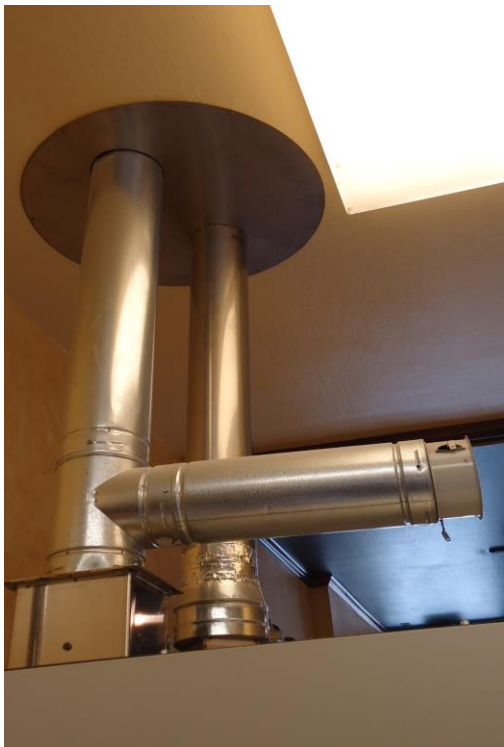
Example of gas exhaust with barometric damper. (See schematics for alternative layouts.)
