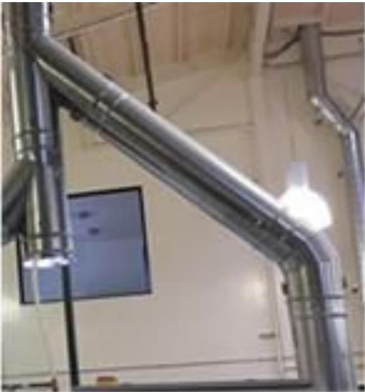
Two steam vents tied together with condensate trap at base. Condensate hose runs to floor sink.
